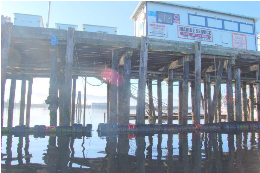
Approach Trestle Bents 13 to 16 (Photo #314) No damage noted, remove debris inside between Bents 14 & 15
