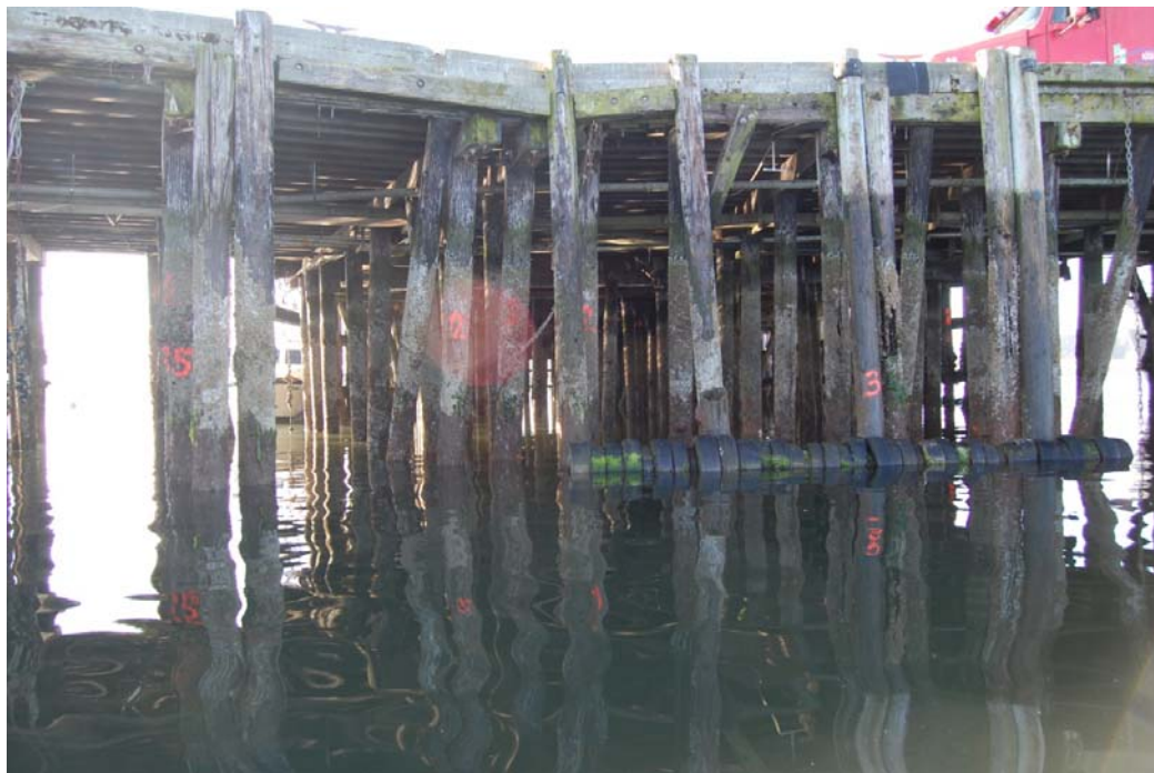
End of Approach Trestle (at left) and the start of the West Wharf (Photo #321) 36"± vertical crack on pile at Bent 3 (shown behind fender pile painted "3")
