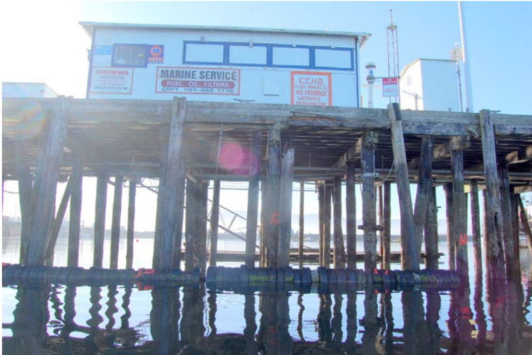
Approach trestle Bents 15 to 18 (Photo #316) Replace broken fender pile at Bent 16
