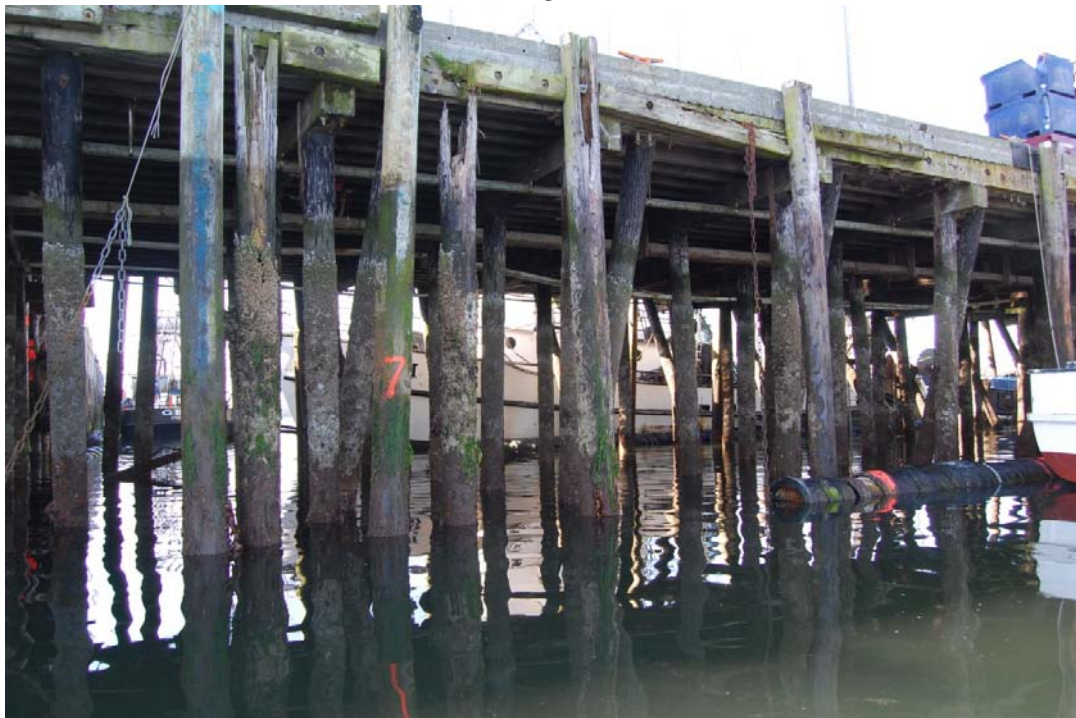
West Wharf Bents 7 to 10 (Photo #324) Repair/replace chock between Bents 8 & 9
