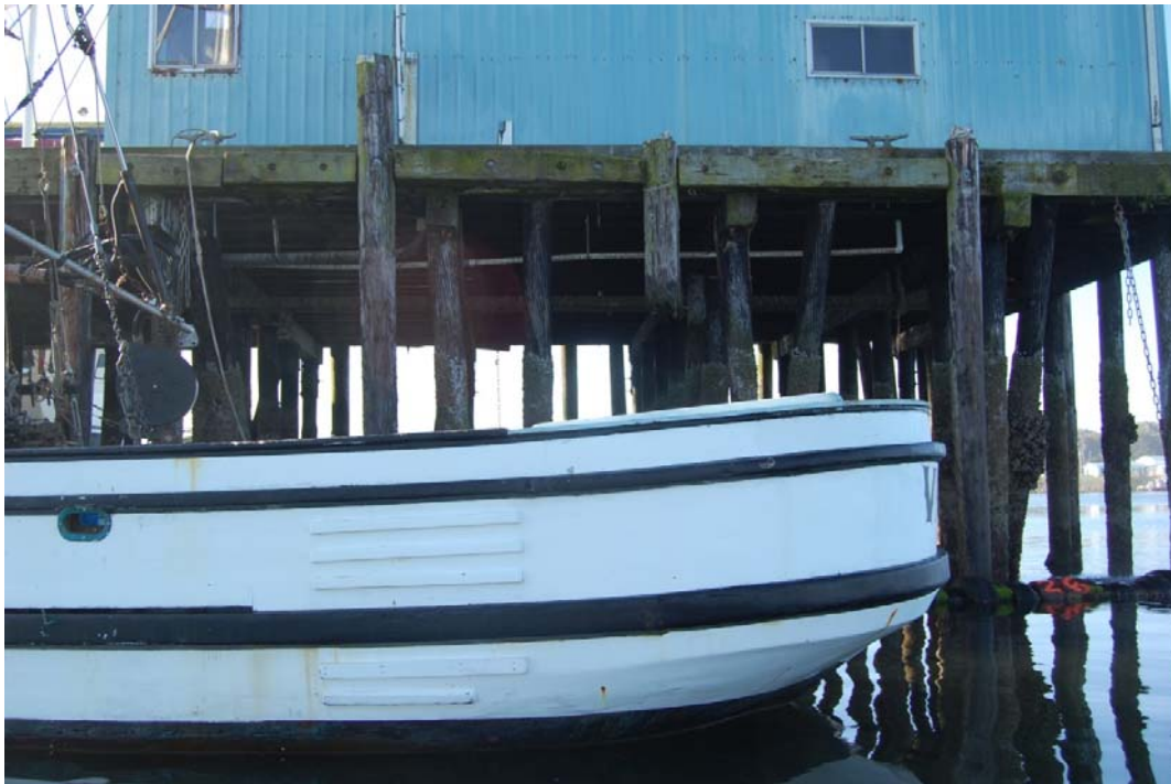
Between Bents 18 and 25 unable to survey due to the vessel "Victory" (Photo #332) Lower portion of fender pile between Bents 24 & 25 is broken off
