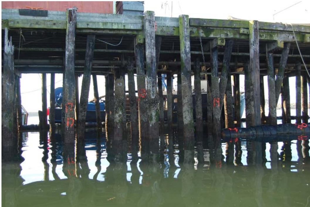
West Wharf Bents 17 to 20 (Photo # 330) No damage noted. Replace missing chock between bents 18 & 19
