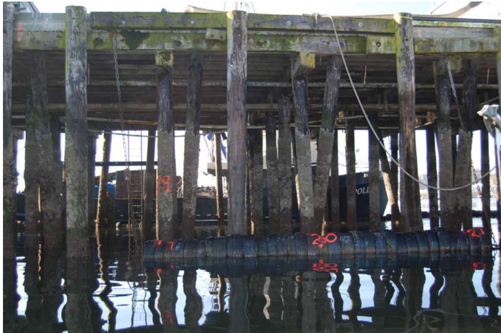
West Wharf Bents 19 to 21 (Photo #331) No damage noted. Replace missing chocks between Bents 18 & 21
