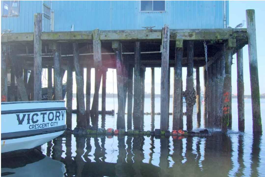
Bents 24 to 27 (Photo #333) Replace broken fender pile between Bents 24 & 25 Add chocks between Bents 26 & 27
