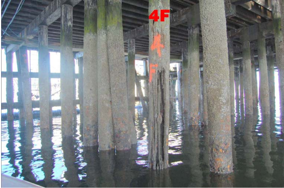
Pile 4F (Photo #371)
