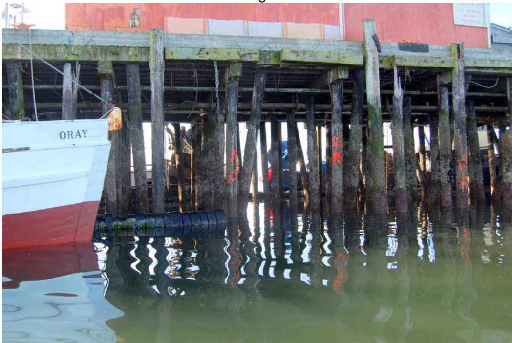
Between Bents 9 and 15 unable to survey due to the vessel "Moray" (Photo #327) Missing fender pile between Bents 15 & 16
