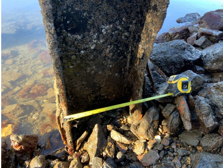
Figure 2-2. Example of steel H-pile (B3) major to severe damage rating
