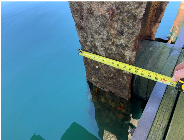
Figure 2-3 Pile A1 with major damage rating
