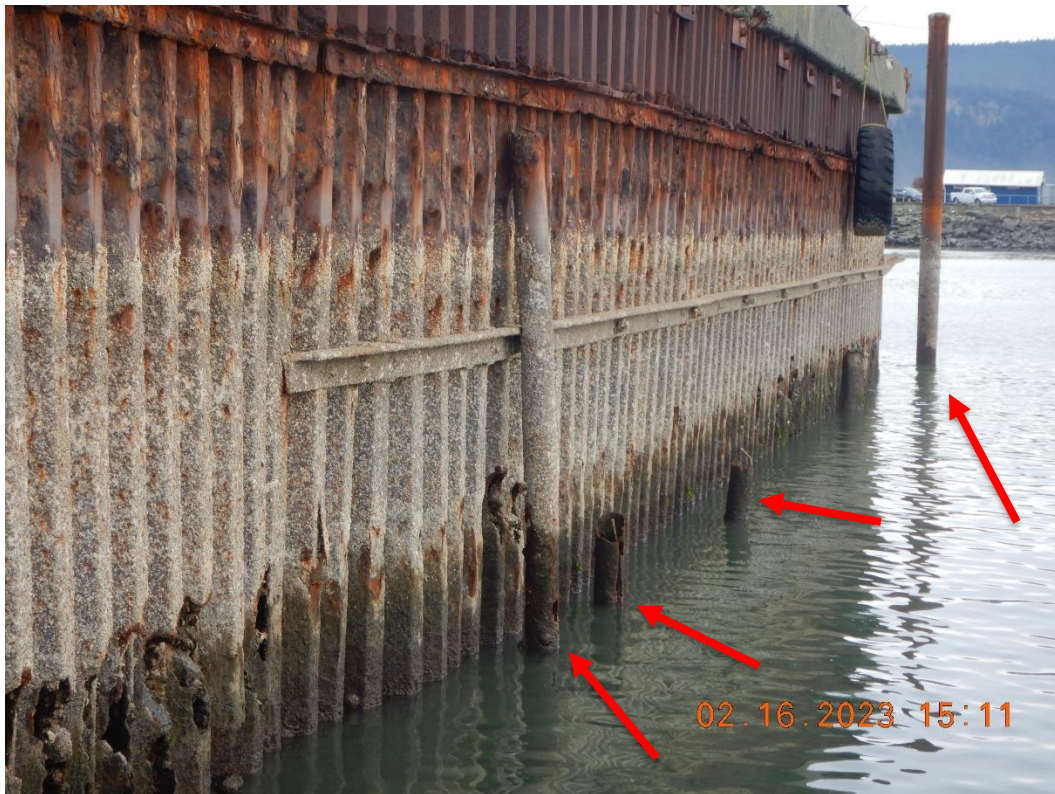
Photo 12. Typical broken fender pile remaining along bulkhead
