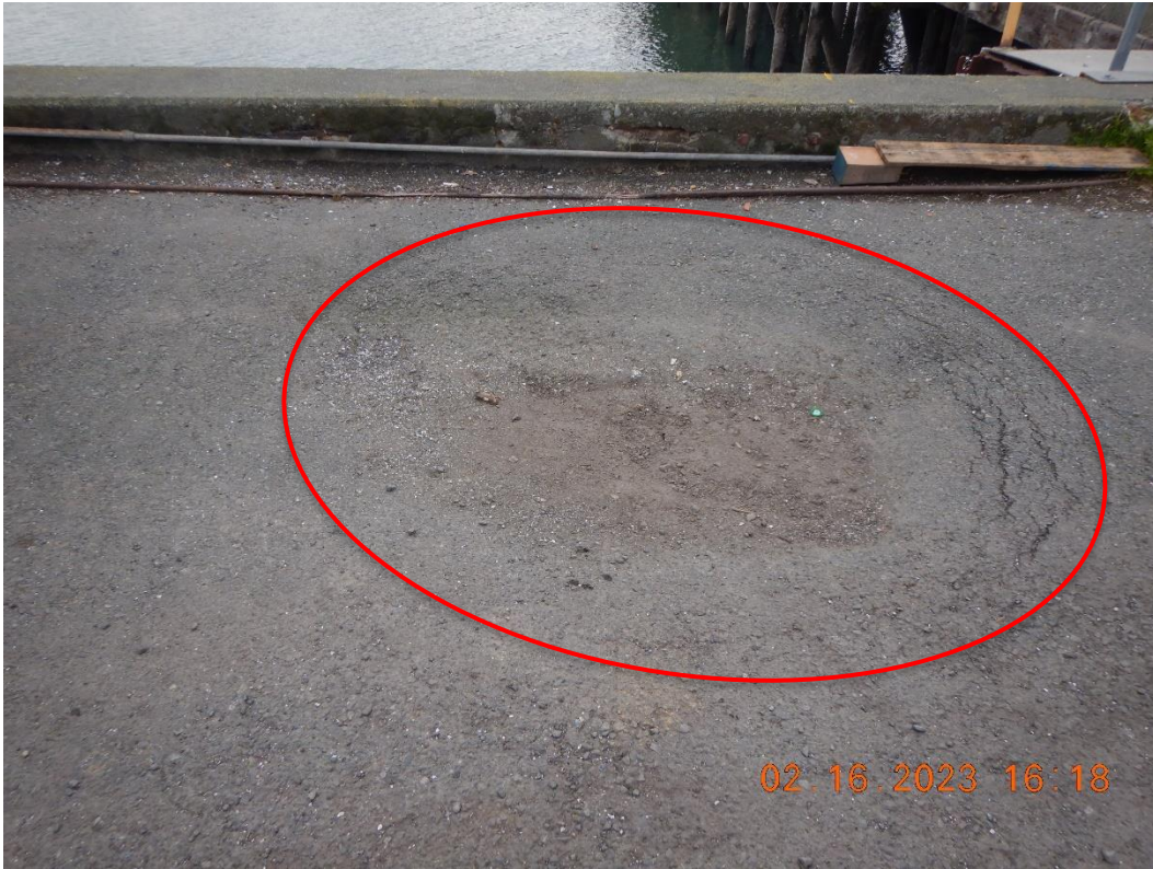
Photo 17. Moderate sinkhole in asphalt paving at STA 0+12
