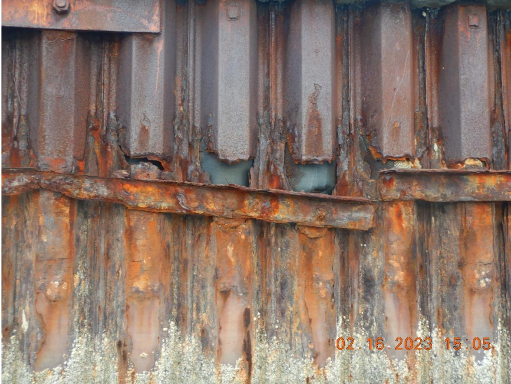
Photo 5. Severe corrosion of upper waler at STA 1+60
