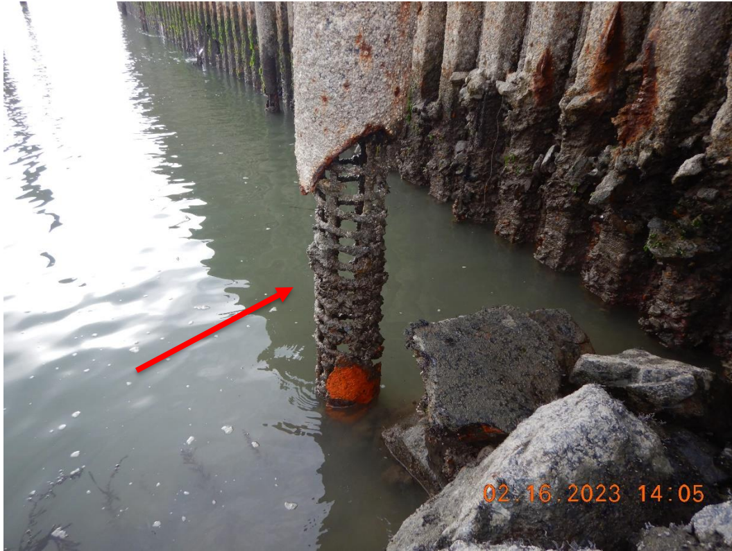
Photo 11. Severe corrosion at platform support pile at STA 3+00
