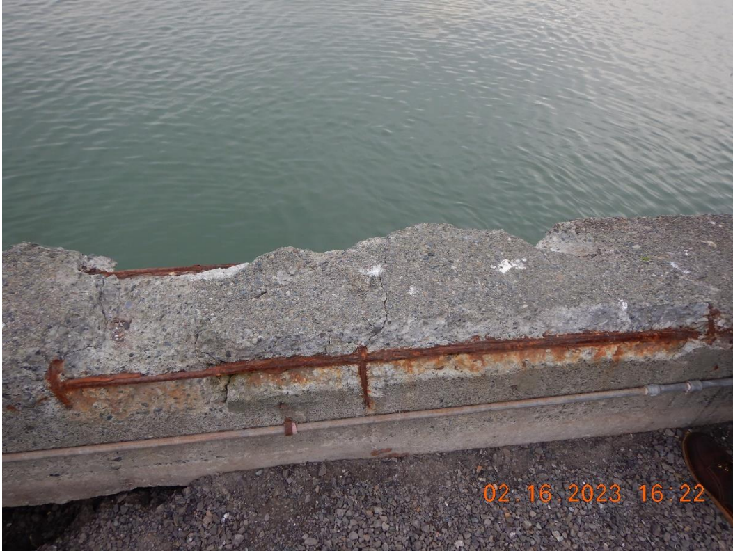
Photo 15. Severe OCS with exposed and corroding reinforcement from STA 1+70 to 1+90
