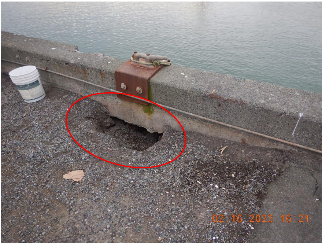
Photo 18. Severe sinkhole at STA 1+73
