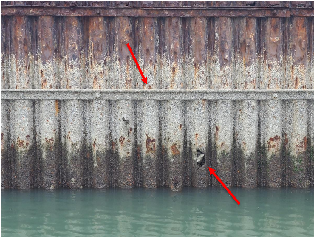
Photo 10. Typical corrosion holes and lower waler from STA 2+00 to 3+00
