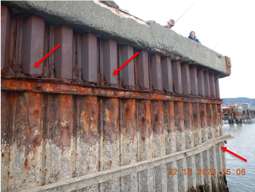
Photo 7. Bent and disconnected lower waler at STA 2+00; typical severe corrosion above upper waler from STA 1+00 to 2+00
