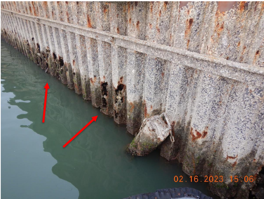
Photo 6. Typical severe corrosion holes and lower waler from STA 1+00 to 2+00
