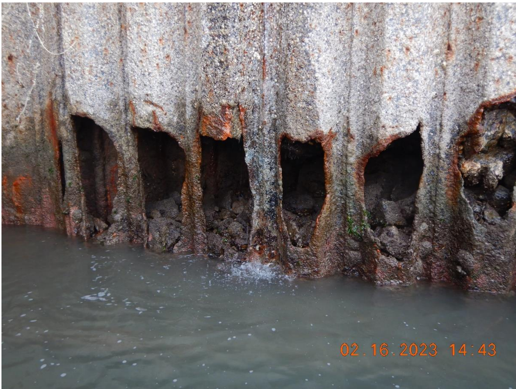
Photo 2. Severe corrosion holes from STA 0+00 to 1+00
