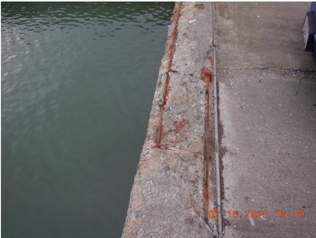
Photo 14. Severe open corrosion spalling (OCS) with exposed and corroding reinforcement from STA 0+43 to 0+70
