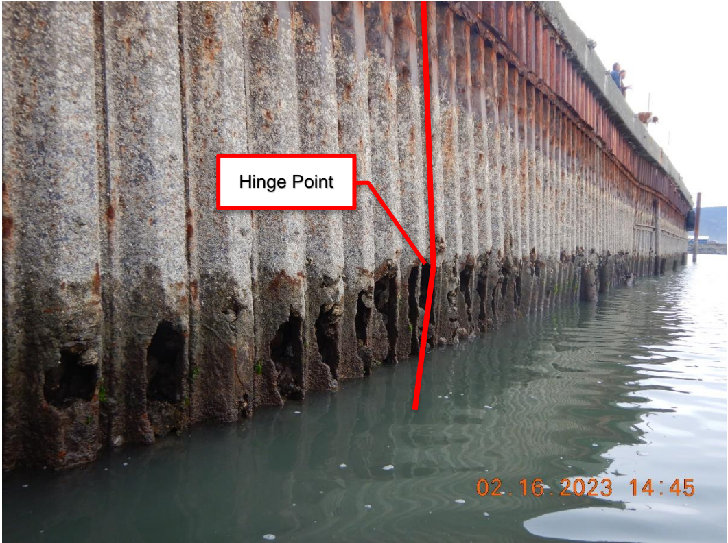
Photo 3. Buckling of bulkhead from STA 0+00 to 1+00
