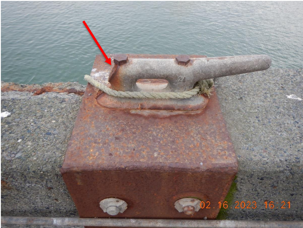
Photo 16. Broken mooring cleat horn at STA 1+73
