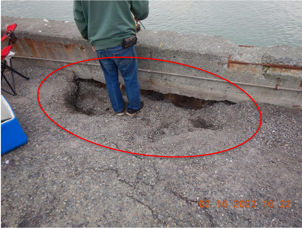
Photo 19. Severe sinkhole at STA 1+90
